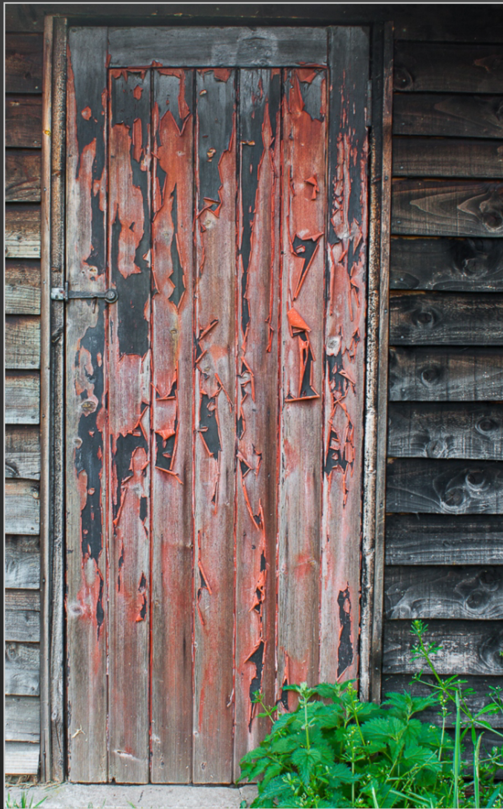
PEELING PAINT by Peter Davis PIC 6
